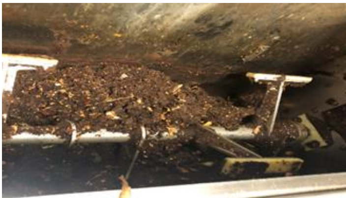
Figure 105 Processing food waste inside the digester
